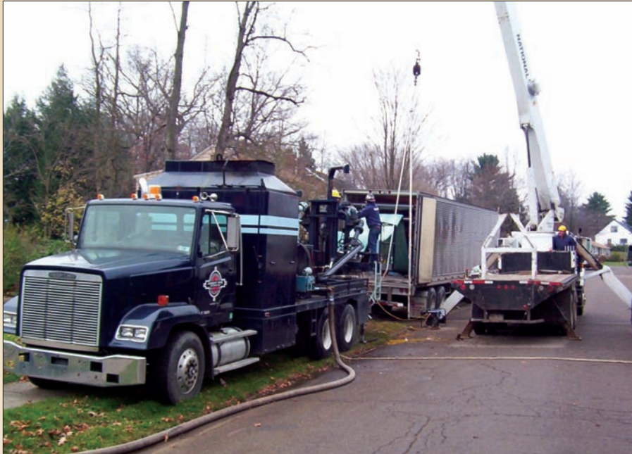
Malcom Pirnie and the City of Oil City, Pa., decided that the best alternative to rehabilitate the Cowell Avenue storm sewer was to install a cured-in-place pipe liner. Three storm sewers of 24-, 30- and 36-in. diameters were CIPP lined.
